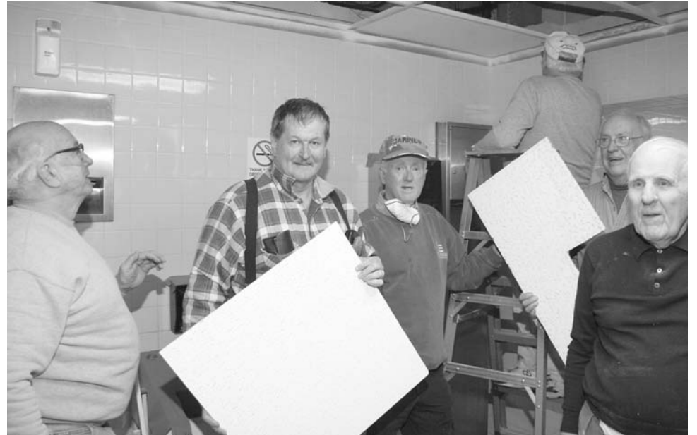
THE VOLUNTEERS CLEANED and painted all the tracking, then installed all new ceiling tiles in the mens and ladies' rooms.
